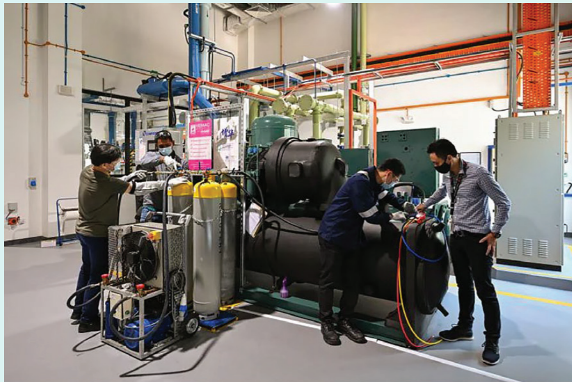
FIGURE 6. TRAINING FACILITIES FOR THE 'REFRIGERANT HANDLING FOR CHILLER' COURSE AT TP
